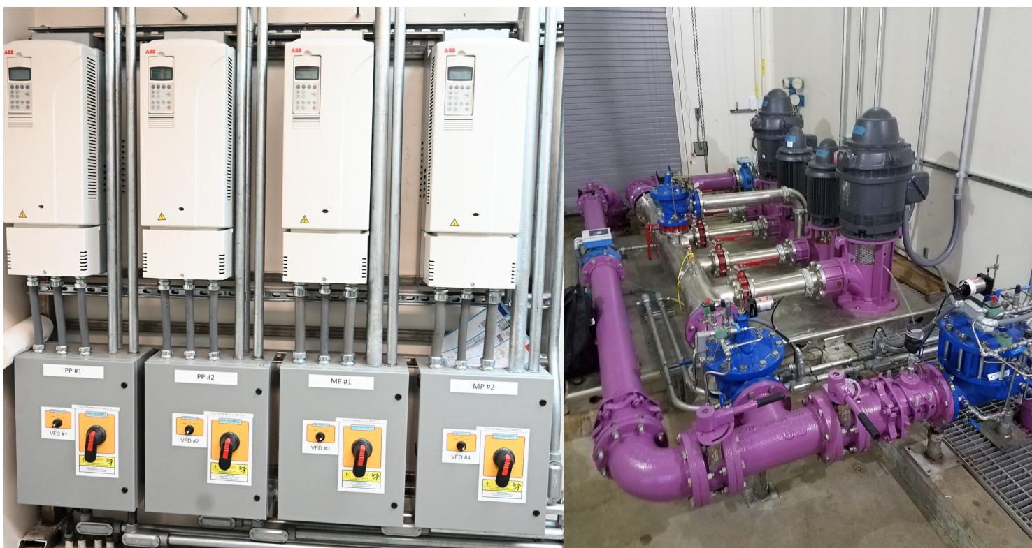
One of the latest upgrades include new Variable Frequency Drives which control the pumps on the water reuse skid shown in the picture to the right.
